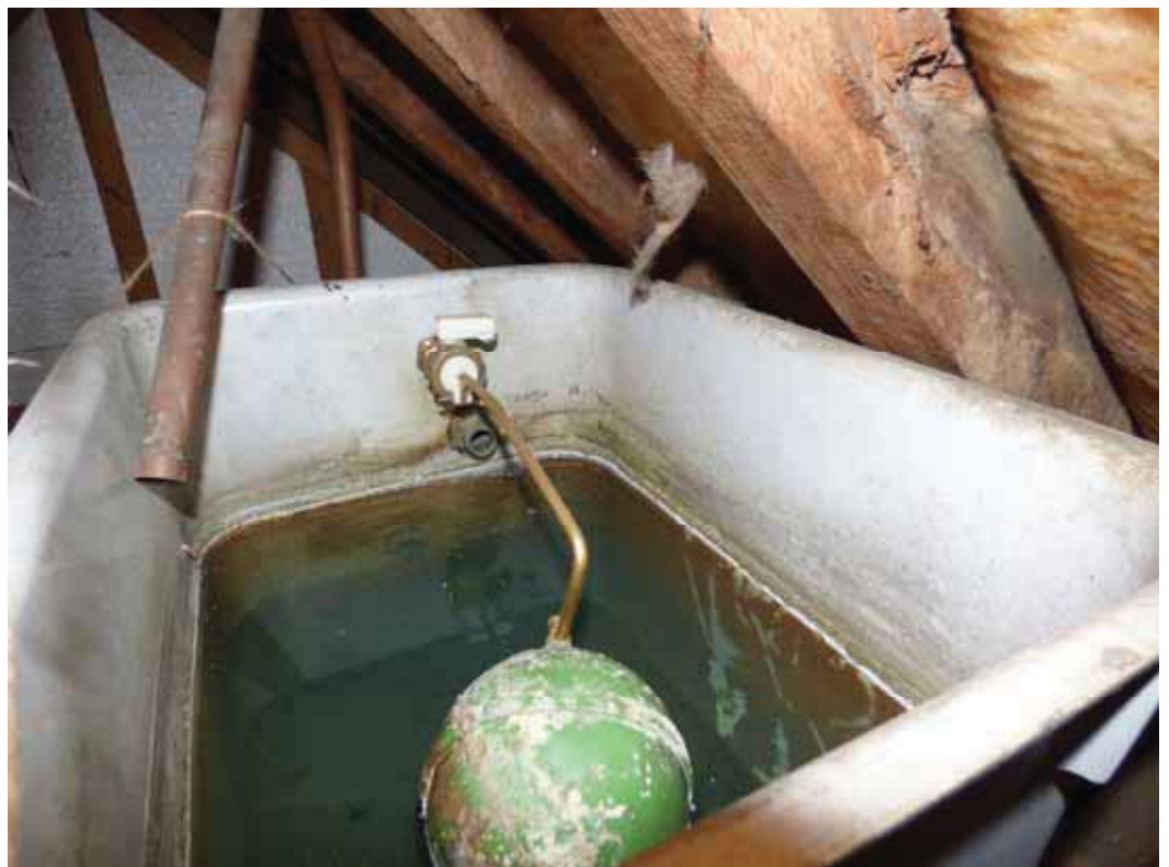
The expansion tank.
