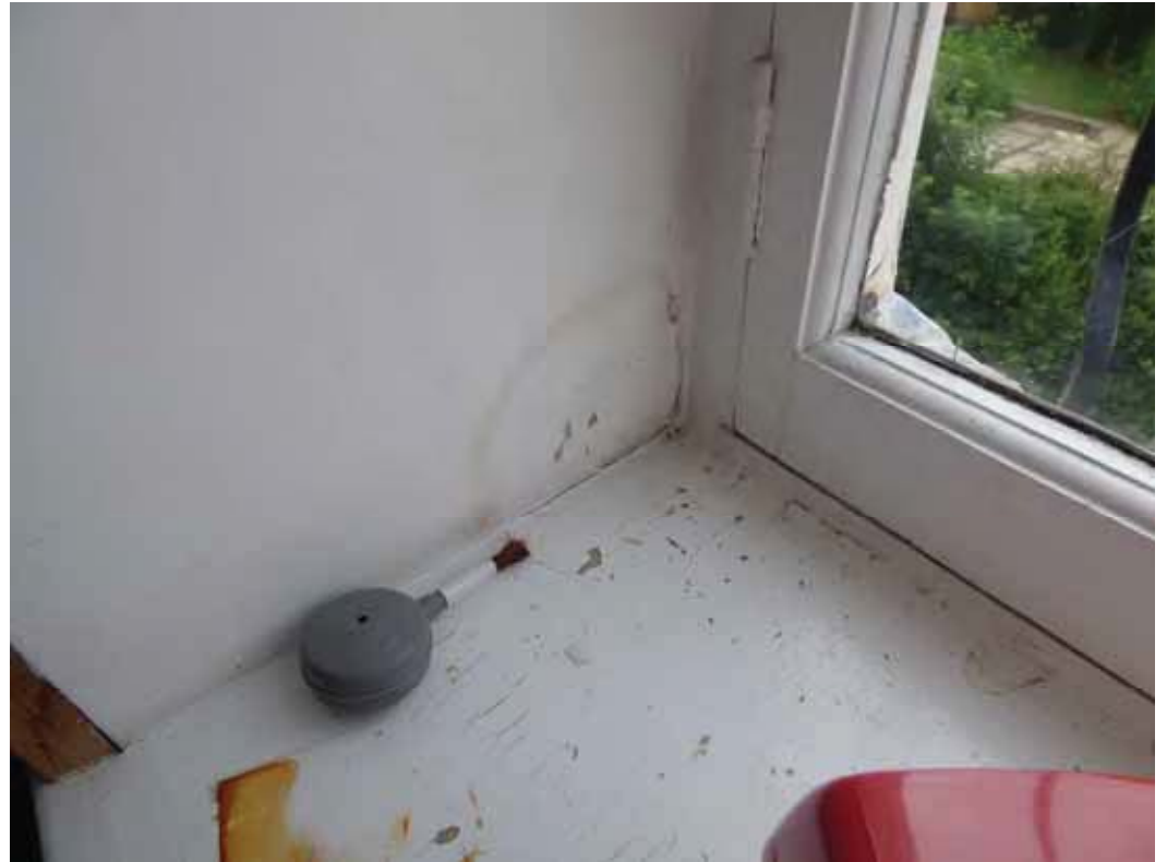
Repairs will be needed to minimise further problems and limit damp penetration.
