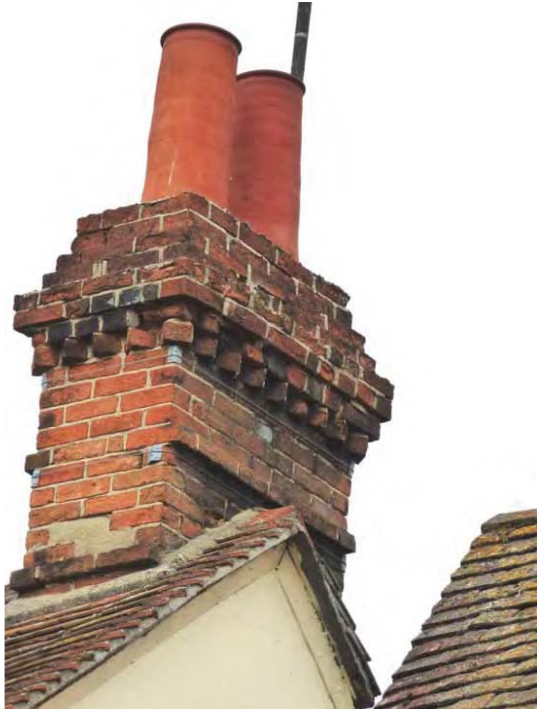
The right side stack, which serves the fireplaces in the first floor sitting room and dining room. The chimney has a more 'fancy' design and is possibly original.
