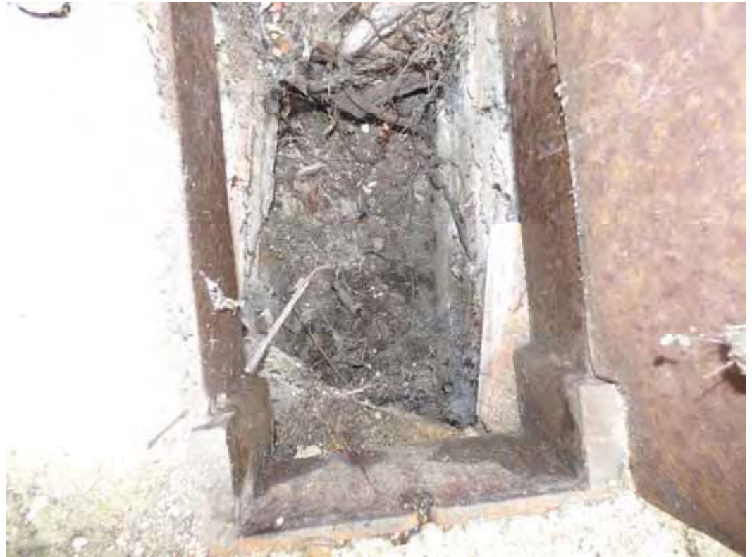
Internal view - there is no meter fitted.
