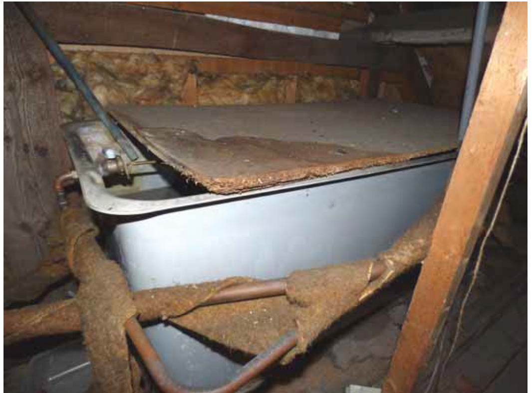
The cold water storage tank – note the poor cover.
