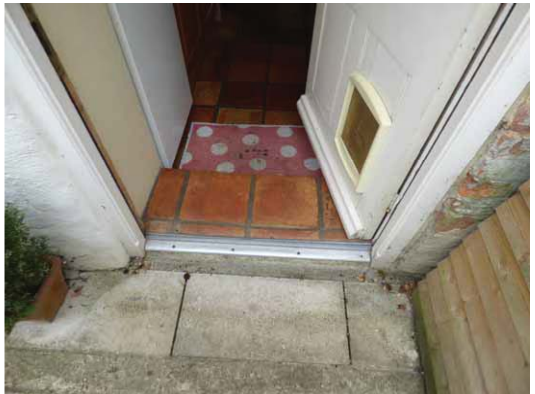
The modern kitchen door – note the high external ground levels.
