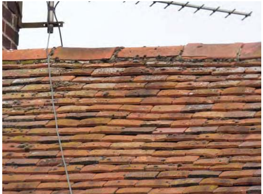
The ridge tiles are satisfactory, although the mortar bedding the tiles has cracked and weathered in areas. Occasional re-bedding may be needed.
