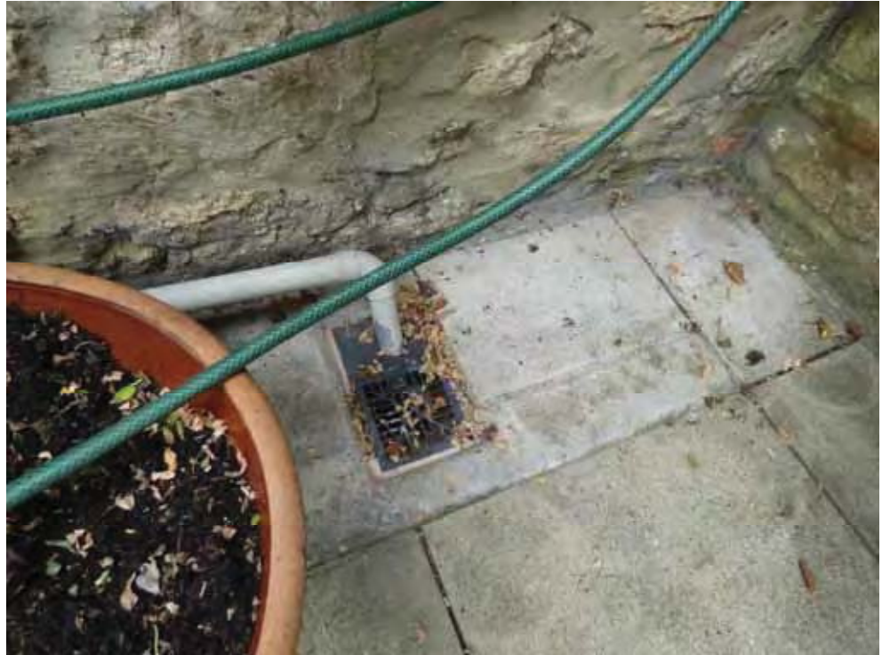
The kitchen gully is satisfactory.
