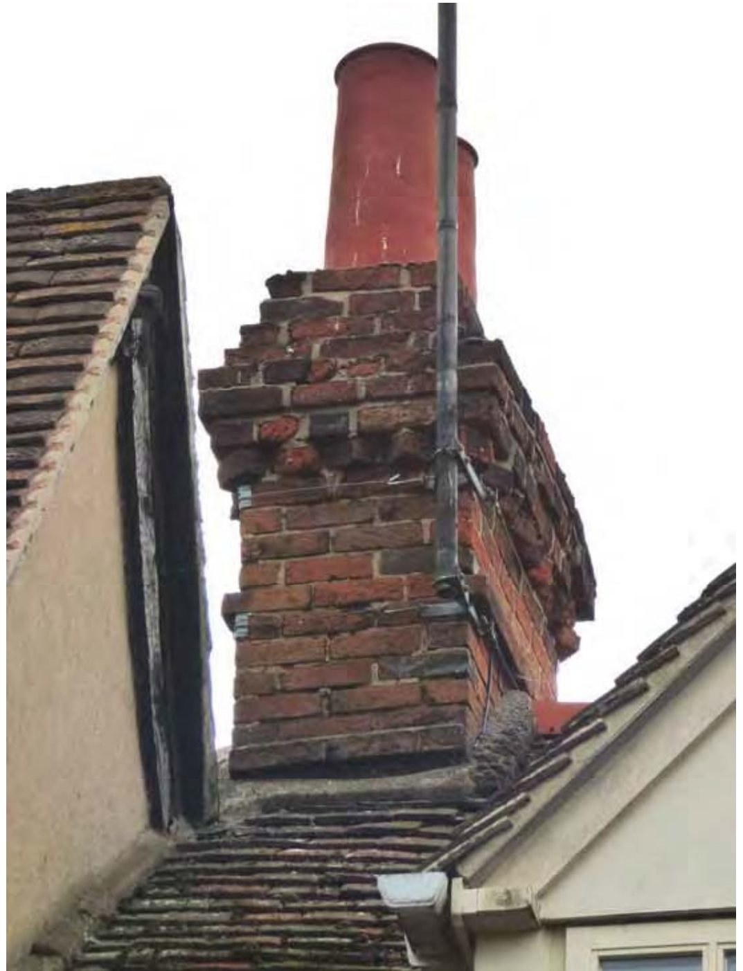
The rear view – note the bulging to the upper courses.
