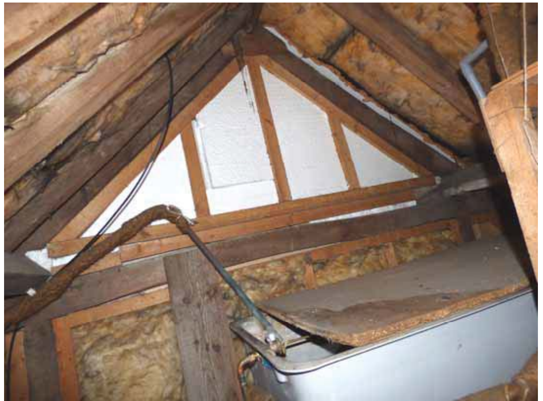
The wall to the right side attic room – this offers limited fire resistance and insulation (although not untypical in an old house).
