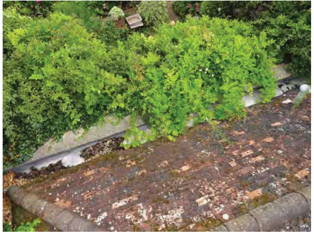
Raised view showing the right side slope and valley gutter. Note the frost damaged tiles.
