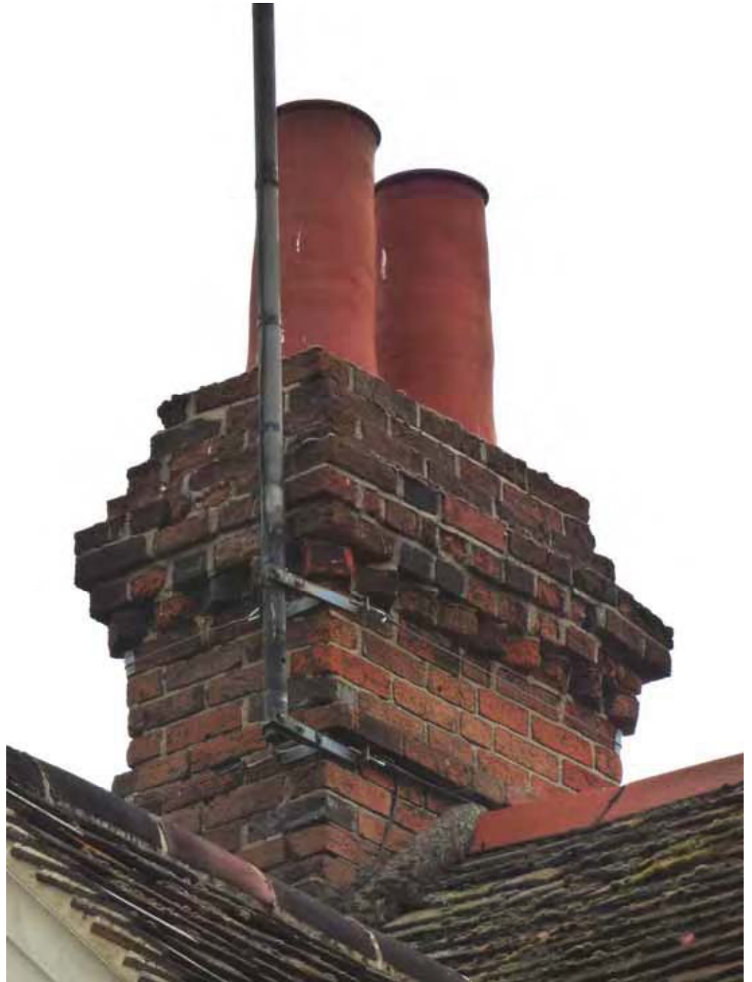
Ditto. Note the weathered pointing to the lower courses of the brickwork.
