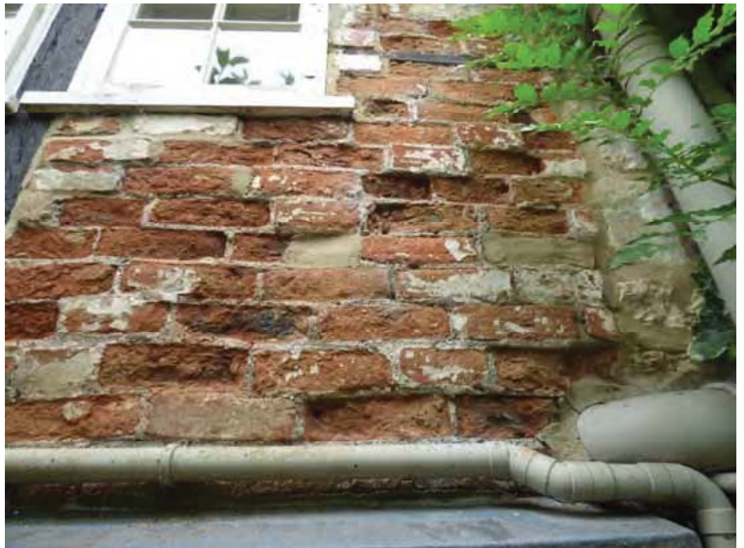
The extensive frost damage to the bricks is not ideal, but they are relatively sheltered and piecemeal replacement is not ideal. You could consider internal linings when renovation works are being undertaken.
