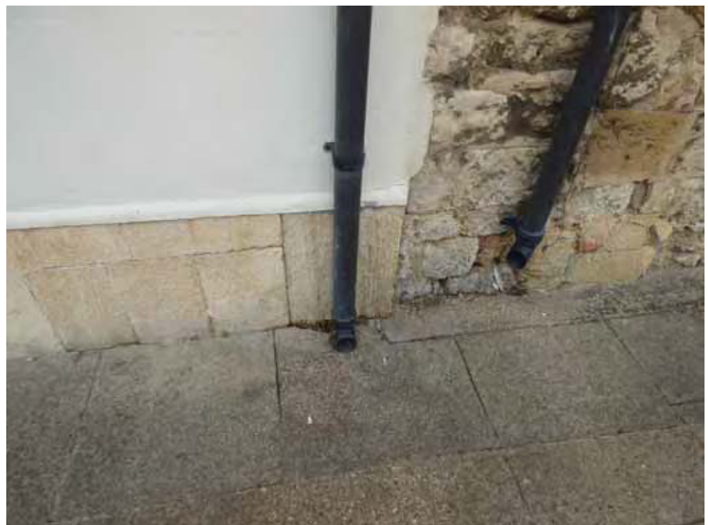
The downpipes at the front spill over the pavement.
