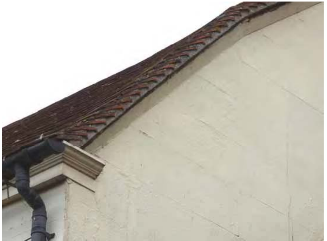
The render will need some general patching, prior to decoration.
