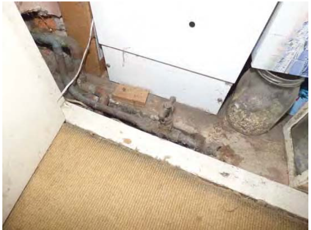
The visible internal stoptap in the understairs cupboard.
