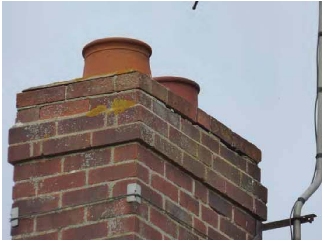
Close view of the upper courses. Note the bricks are lifting.
