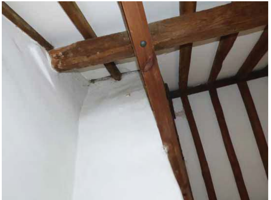
There is less dampness, but the area should be monitored.
