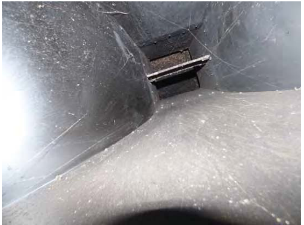
Internal view of the smoke hood.
