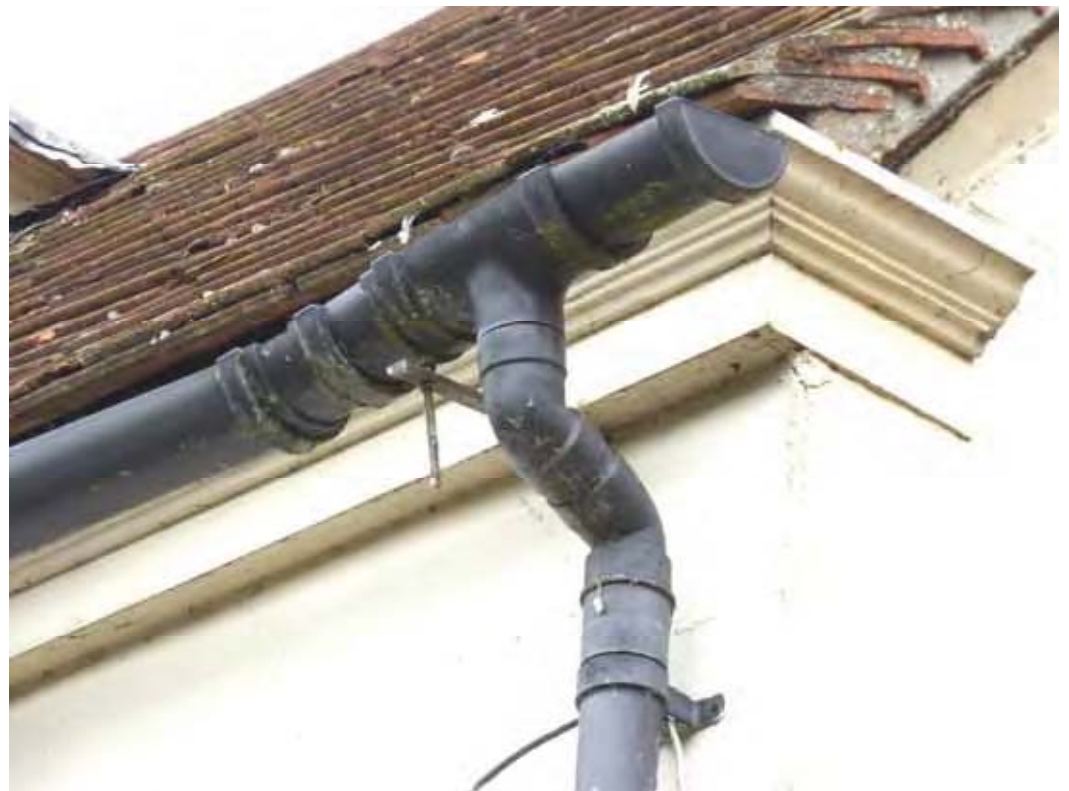
The front right side stop end is out of alignment.
