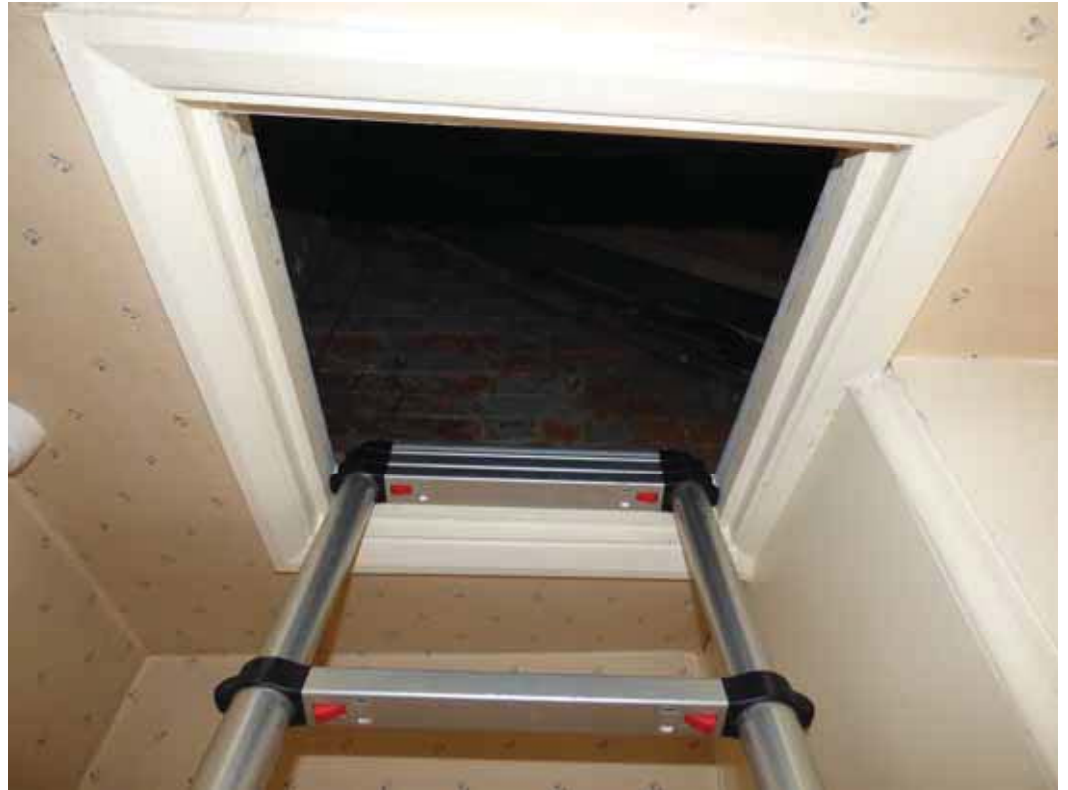
There is also a good hatch into the eaves area over the bathroom.
