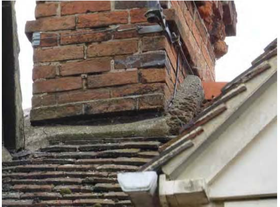
The fillet is slightly cracked.
