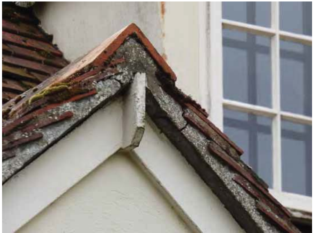
The mortar to the verges has cracked and weathered. Occasional patch pointing will be needed.
