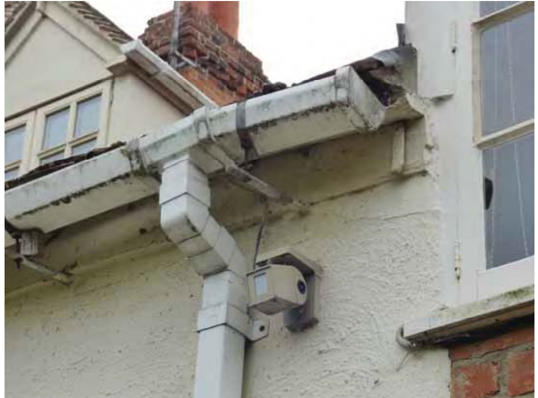
The gutters are also misaligned in areas.
