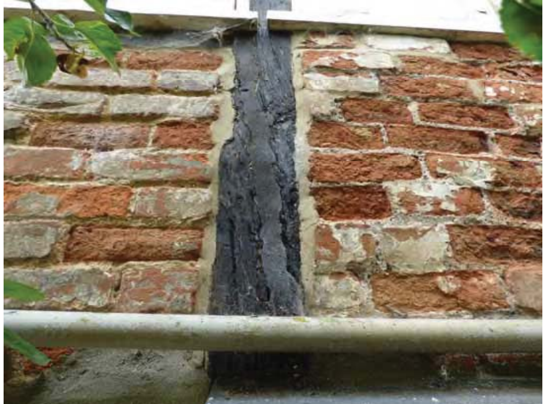
The filling of the timbers will mortar should be avoided, if possible. They are also best left unpainted.
