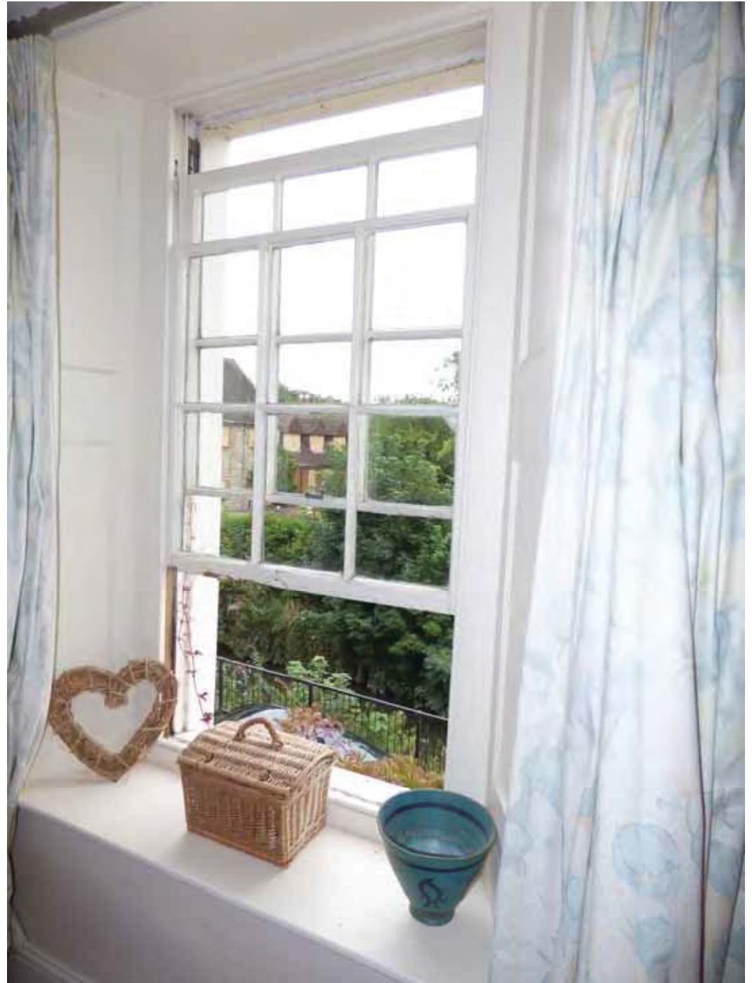
Note the rot to the lower sash – these windows are made with good quality timber, but lack of maintenance has allowed some decay, which will need repair.
