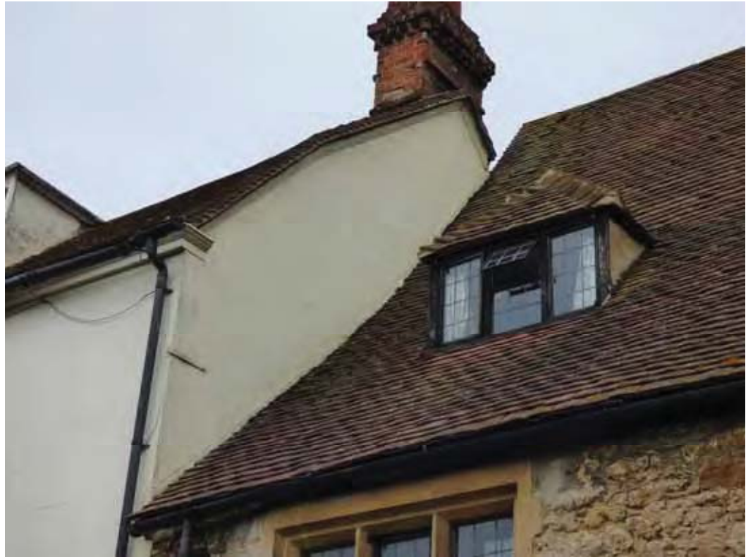
The right side gable has been painted and there are no signs of movement.
