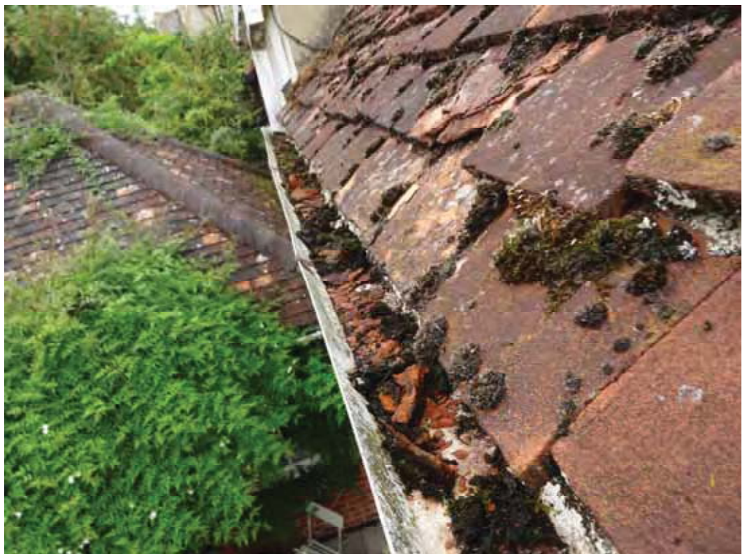
Regular cleaning will be needed due to moss, creepers and the frost damage to the tiles.
