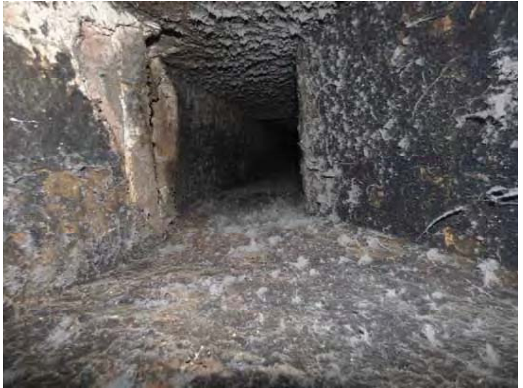
Internal view of the flue. The cobwebs indicate that the flue appears to have been little used recently.
