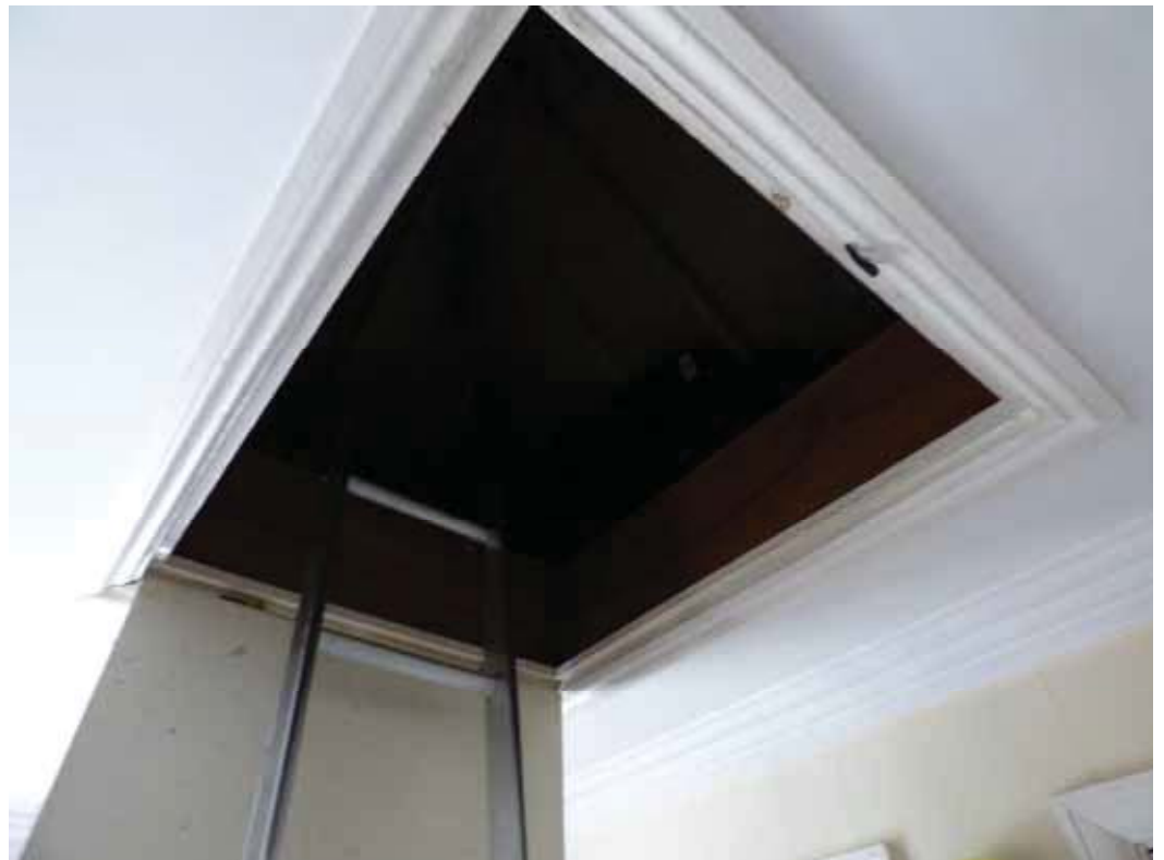
The hatch into the extension roof – there is a light and loft ladder (although this is broken).
