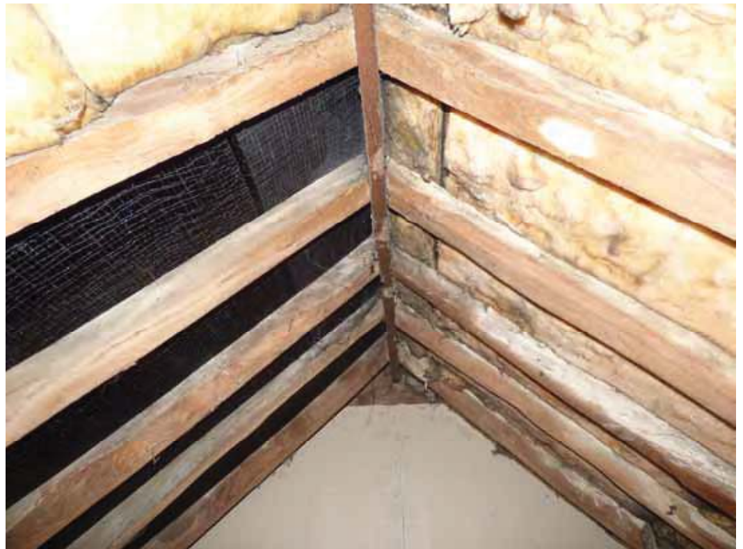
The timbers are built to a ridge board indicating they are likely to be nineteenth century, rather than earlier.
