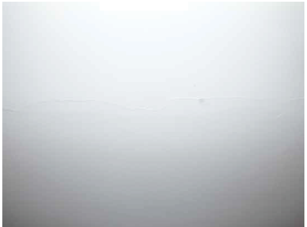
Typical shrinkage cracking to the plasterboard ceilings.
