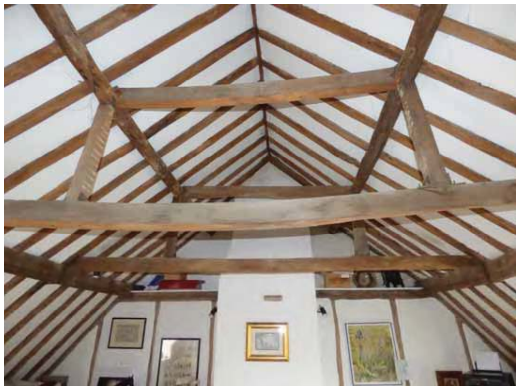
The left side area as visible in the attic room – view left.
