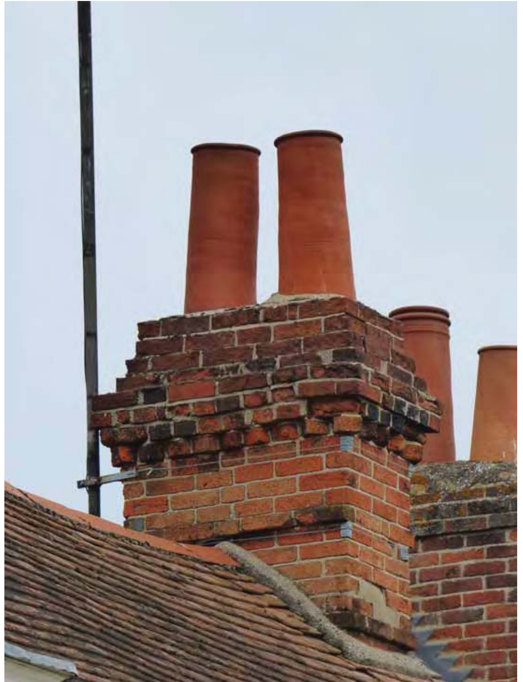
The front left side view – note the pots are out of true and there is cracking visible to the bedding mortar. There is a risk of falling masonry and they should be checked and re-bedded, as necessary. The mortar fillets are in better condition.
