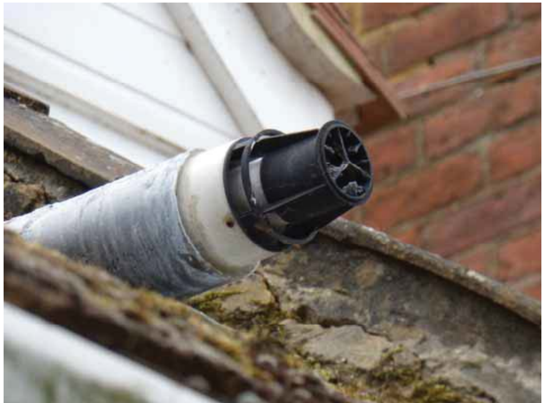
The newer combi boiler and flue.
