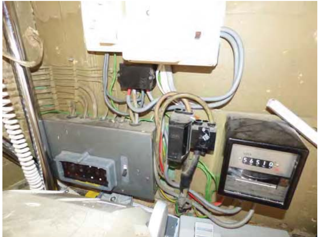
The meter and consumer units. The installation is dated and will need updating.
