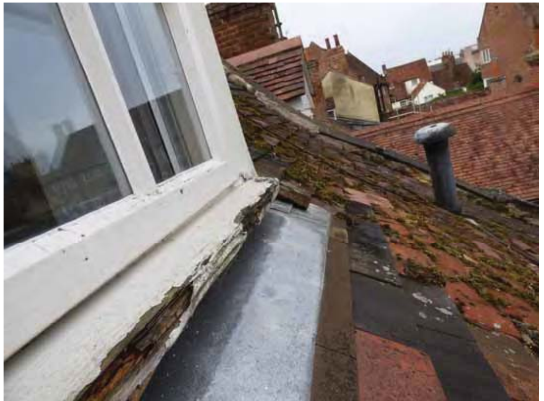
There is considerable decay.
