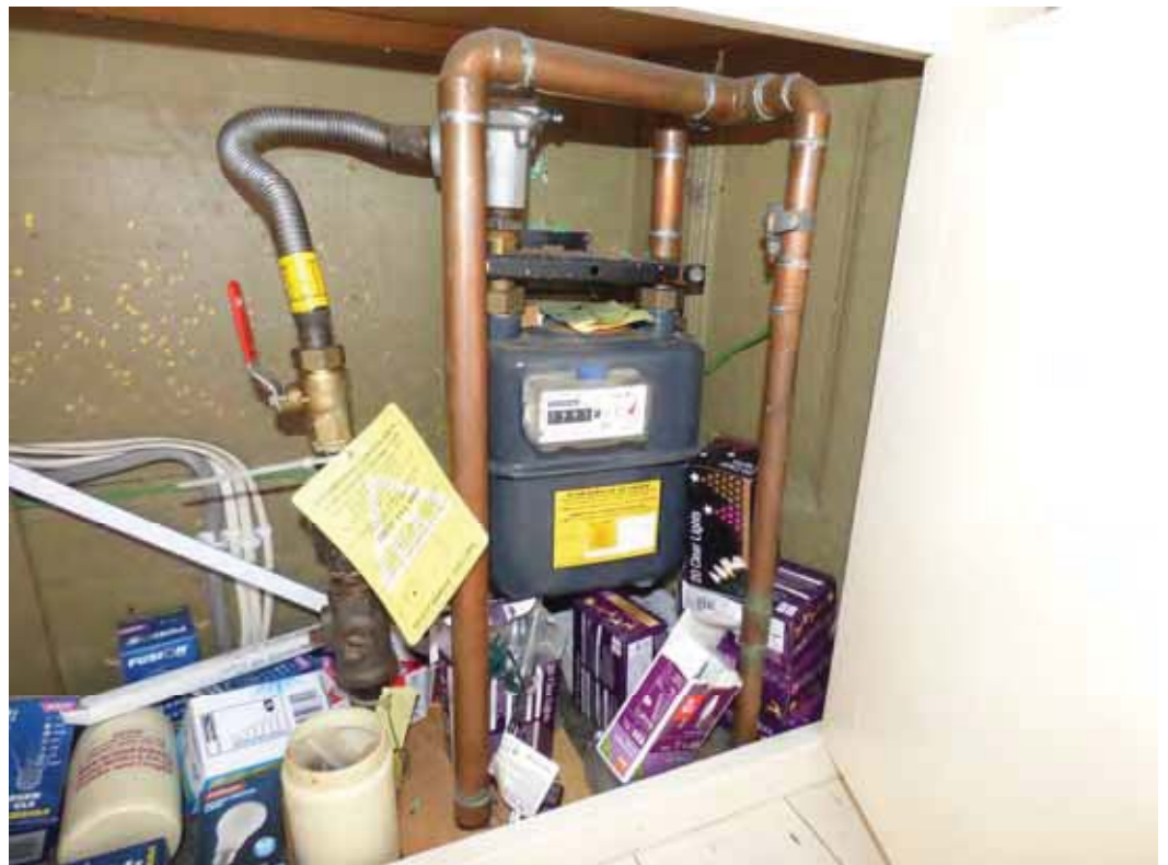
The gas meter.
