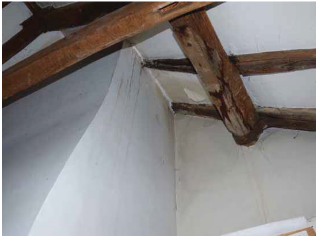
The chimney breast and damp penetration in the attic bedroom below.
