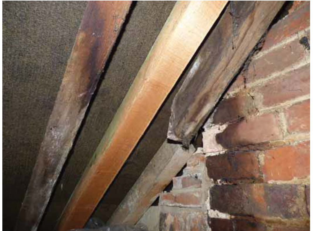
View right – some of the rafters are charred and there may have been a small fire, possibly from the old rear stack.
