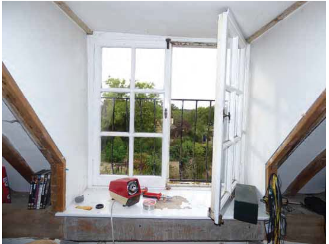
The front frames to the dormers are difficult to access and they have not been maintained.
