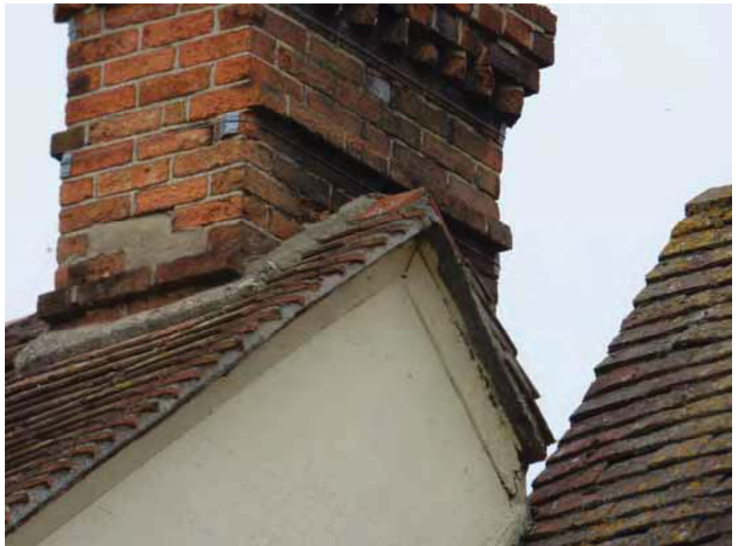
Close views. Note the basic patching to the frost damaged brickwork.
