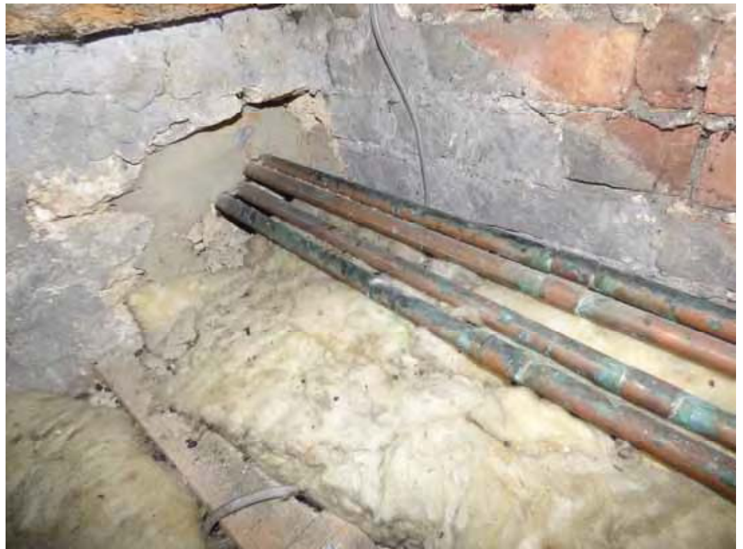
Better insulation is needed to the stud walls, tanks and pipes in the roof void areas.
