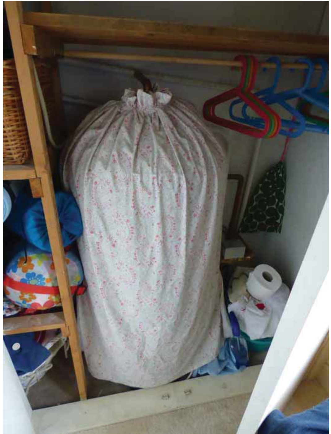
The foam lagged hot water cylinder.
