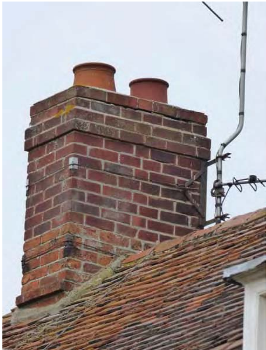
The left side stack, which serves the ground floor sitting room and would have served a fireplace in the bedroom above.
