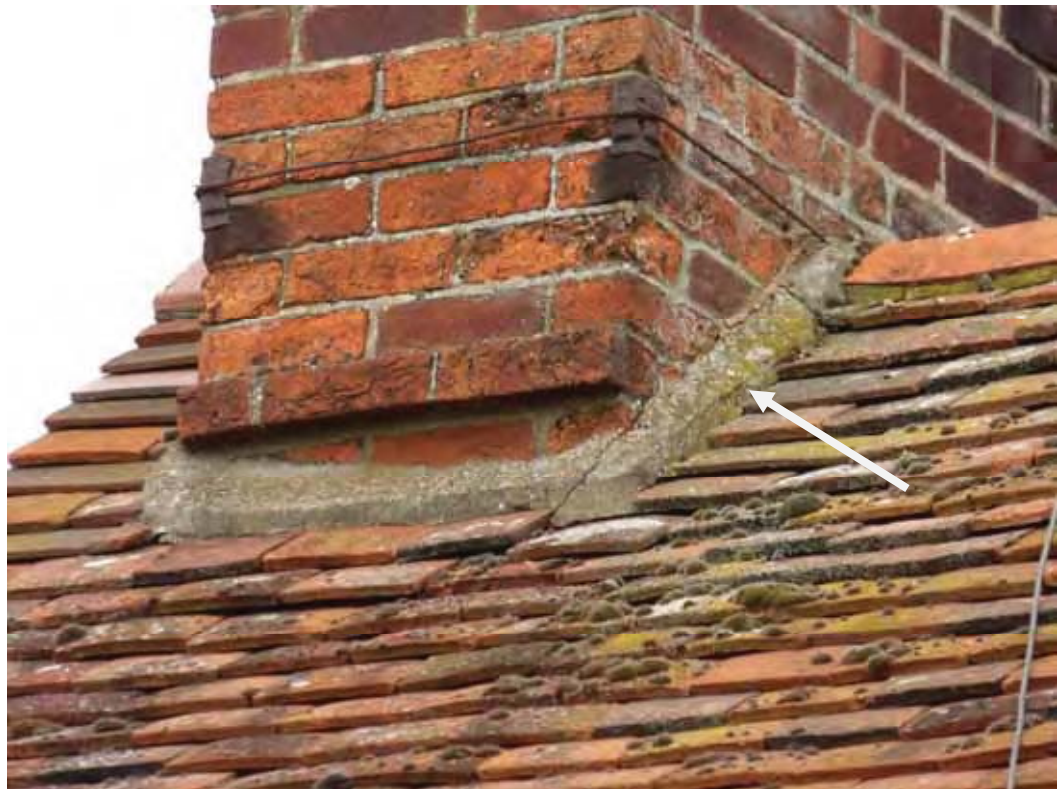
Close view of the mortar fillets – note the cracking and short-term patching with mastic sealer.
